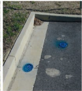
Valve box cover marking
