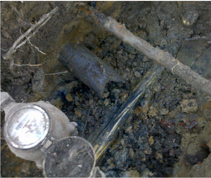
CROSS BORE BEFORE REPAIR
